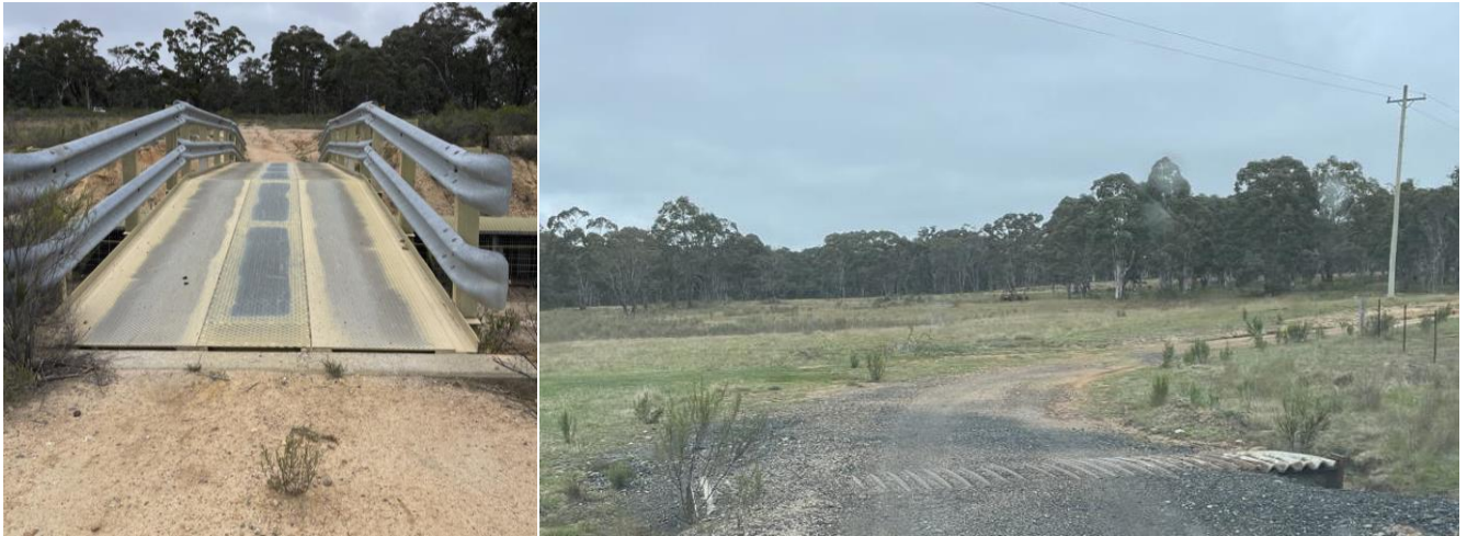
Figure 4.6 Existing structures within access tracks (left: bridge over conveyor belt; right: farm culvert along access point 3)
