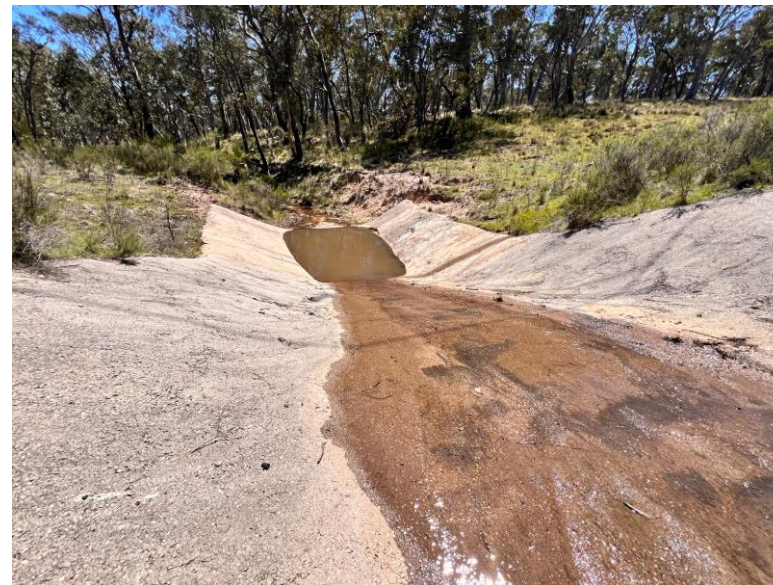
Concrete drop structure downstream of existing transmission line easement, facing north-east (downstream)
