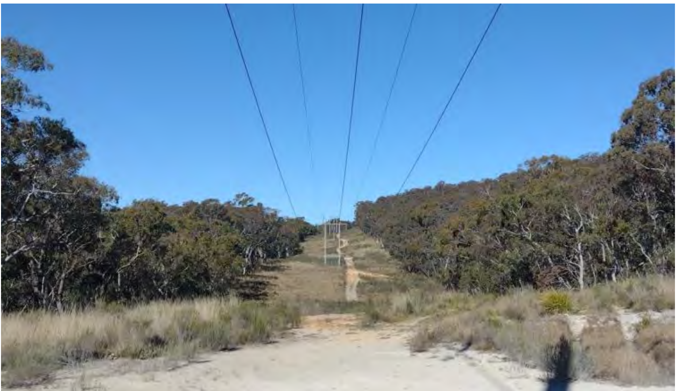
Figure 4 Existing maintenance track along the easement of the 132 kV Line 94E, showing timber 'H' support poles
