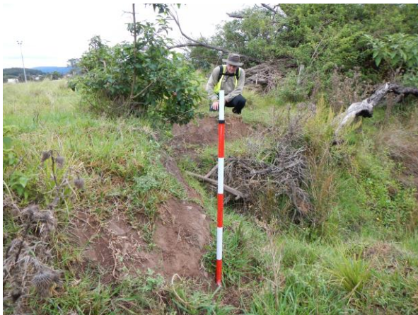
Plate 9: Survey Unit 3 – erosion along the western bank of Frazers Creek, view to NW.
