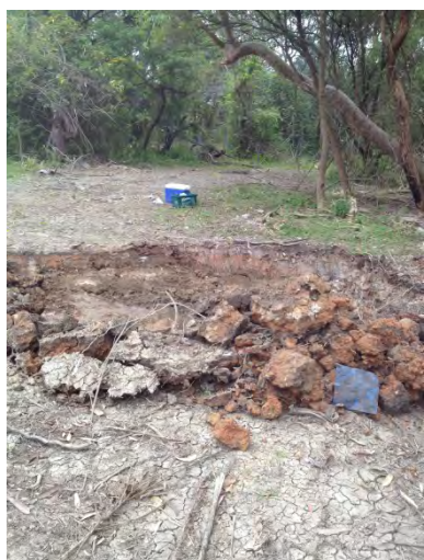
Photo 9 – TP53 where rubbish in fill below a thin clay covering was encountered. Photo looking northeast towards heritage zone
