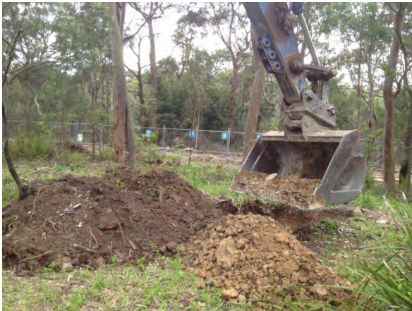
Photo 15 – Spoil excavated from TP61 showing C&D waste
