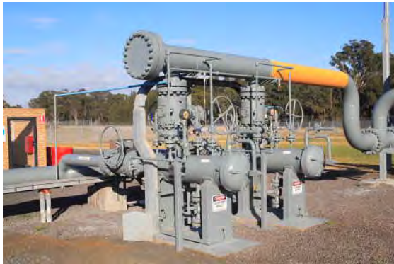
Plate 1-3 Dry gas filters and associated pipework
