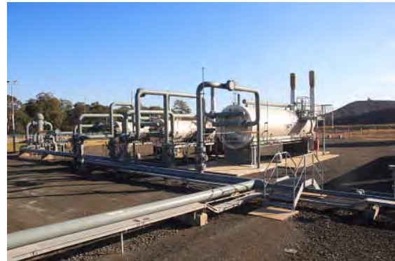
Plate 1-4 Water bath heaters (three) and associated pipework
