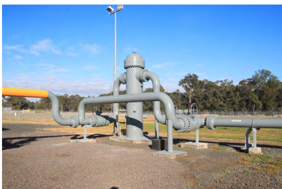
Plate 1-5 Bulk liquid separator and associated pipework
