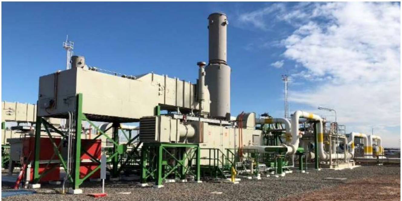
Figure 3.2 Compressor station and vent stack example
