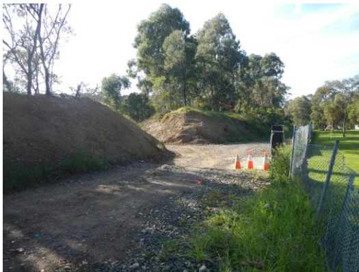
Figure 4: View to the East, showing cuttings to construct access tracks within the road reserve.
