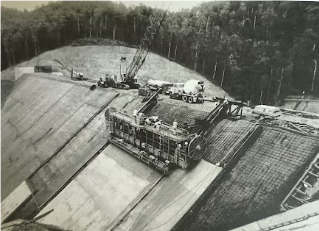
Plate 3.10 The giant screed machine applying a 300 mm concrete face to the inner compacted rock fill dam wall (Source: Johansen 2015:81).
