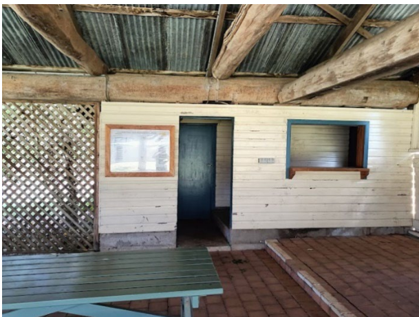
Plate 4.15 Entry to dairy/kitchenette addition. Previous square notch for support post is visible above doorway (Source: EMM 2023).
