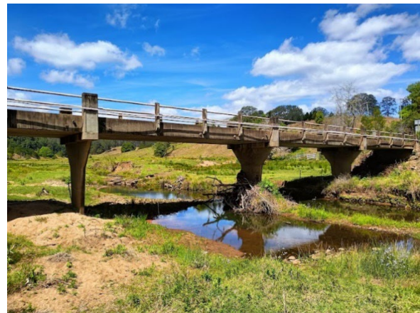
Plate 4.22 Current concrete McCabes Bridge. Former streambed crossing is visible beneath the bridge to the east (Source: EMM).
