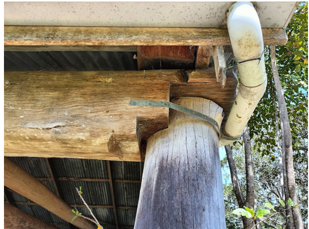
Plate 4.14 Replacement post showing square notched joinery with remnant notching for previous post at base. (Source: EMM 2023)
