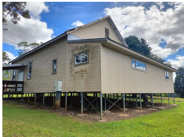
Plate 4.8 Rear skillion addition to Doon Doon Hall on modern steel and concrete supports (Source: EMM 2023)
