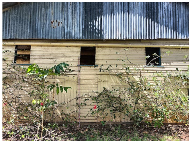
Plate 4.12 Exterior of western end with bail doors visible below windows (Source: EMM 2023).
