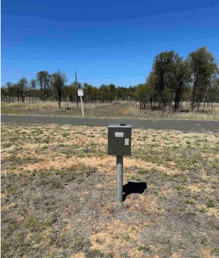
Figure 3.7 Example of a cathodic protection test point
