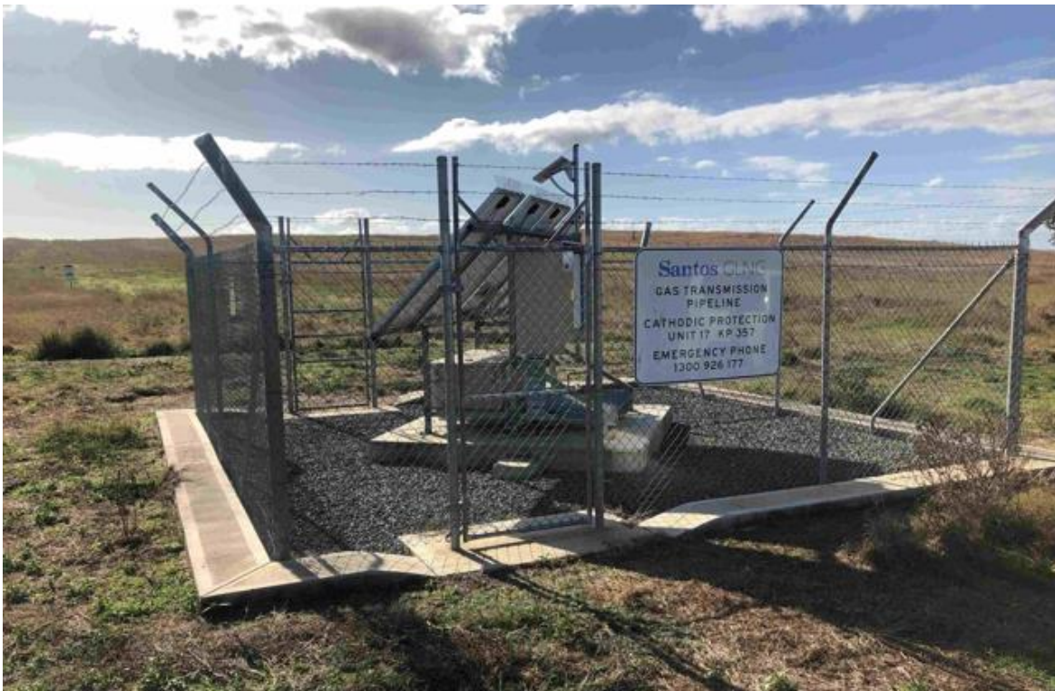
Figure 3.6 Example of a cathodic protection unit (with solar panels)
