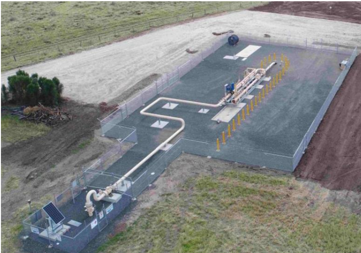
Figure 3.5 Example of a typical scraper station
