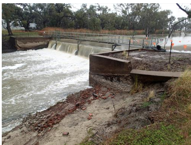
Figure 9.1 Looking upstream at Hartwood Weir at failure of concrete side wall on left hand side of channel
