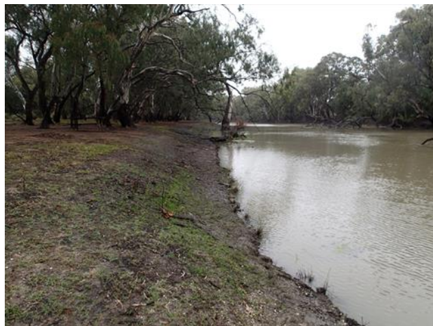
Figure 9.6 Upstream of Wanganella Weir. Minor erosion/notching of banks in weir pool
