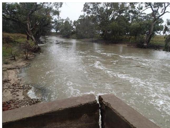
Figure 9.4 Looking downstream of weir, evidence of ongoing erosion of banks and channel widening
