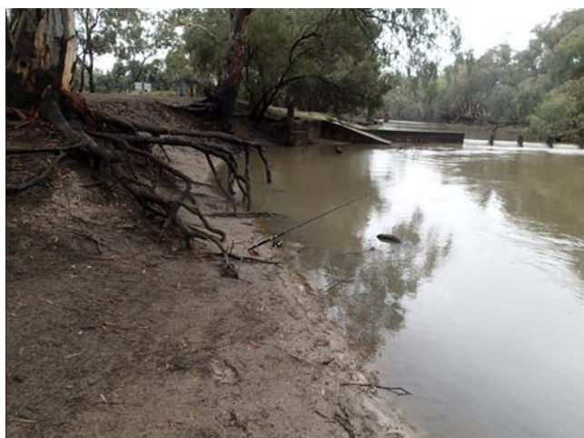
Figure 9.7 Bank erosion downstream of Wanganella Weir
