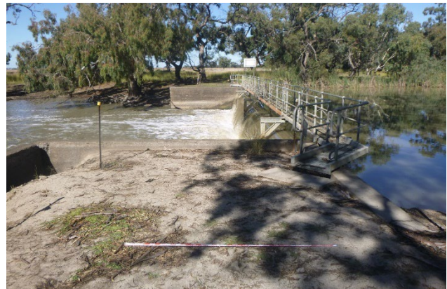
Figure 4-2. Close up view of Hartwood Weir, facing east (Photograph by Brendan Wong)
