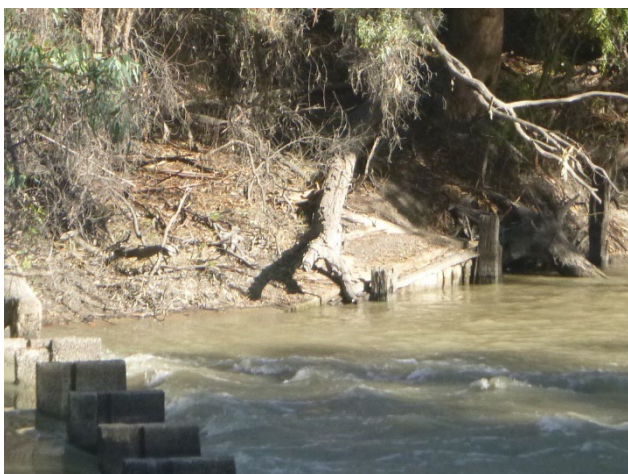
Figure 4-28. Wanganella Weir with timber formwork visible, facing south (Photograph by Brendan Wong)
