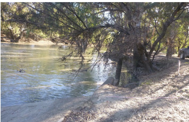
Figure 4-24. Wanganella Weir's ramp and abutment wall, facing west (Photograph by Brendan Wong)
