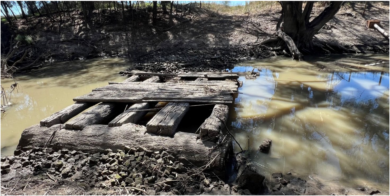
Figure 4-13. Water Group NSW DCCEEW photograph of the Old Bridge, taken on 30 January 2024
