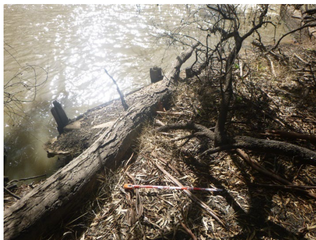
Figure 4-29. Wanganella Weir with timber formwork visible, facing north (Photograph by Brendan Wong)
