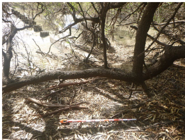
Figure 4-27. View of Wanganella Weir from the south bank, facing northeast (Photograph by Brendan Wong)
