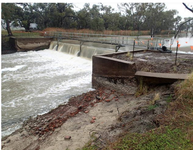
Looking upstream at weir at failure of concrete side wall on left hand side of channel.
