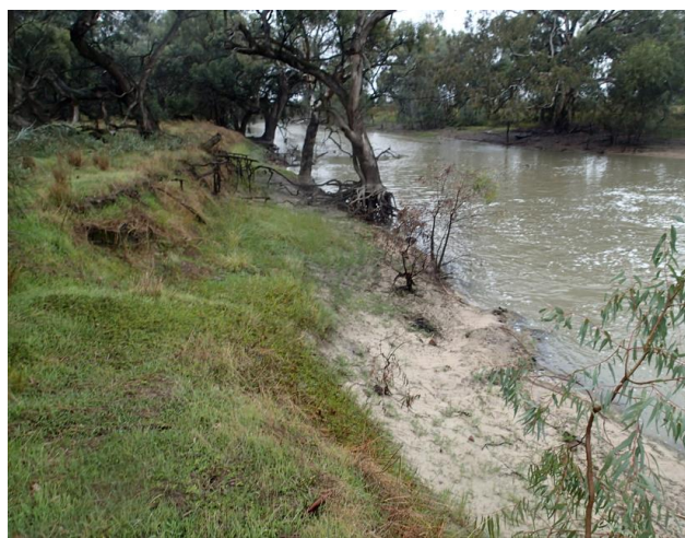
Looking downstream at erosion of channel bank on left hand side of channel.
