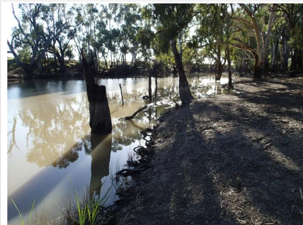
Looking at channel upstream of existing weir. Minor erosion/notching of banks in weir pool.
