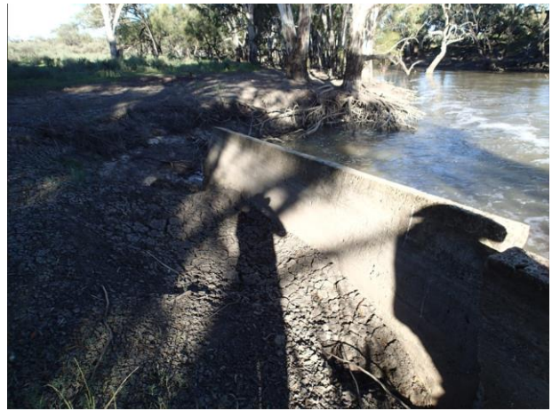
Looking downstream at erosion of channel bank on left hand side of channel.
