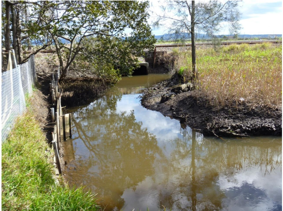
Figure 2-9 Maitland Road Creek bank erosion and retaining wall
