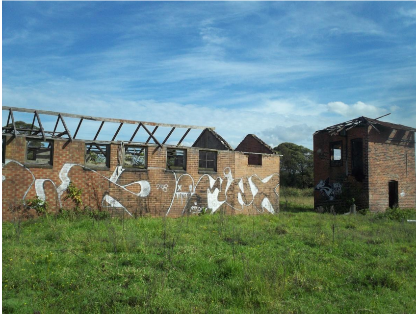
Photograph 10: Dilapidated building near high pressure gas main
