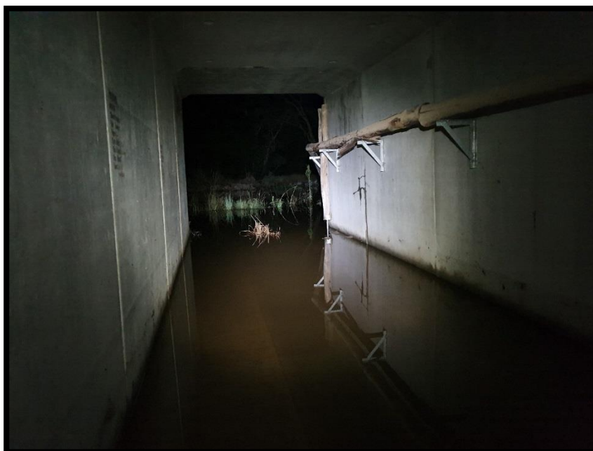
Plate 5-7. Connectivity structure at ch.19180 during surveys on 20 th January 2020 following heavy rainfall.
