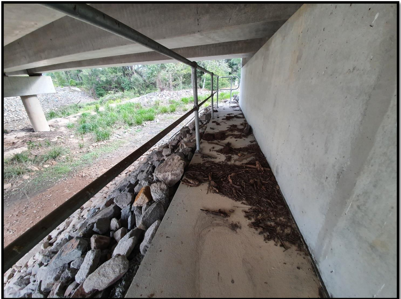
Plate 3-7. Flood debris showing height of flood waters during 2020.
