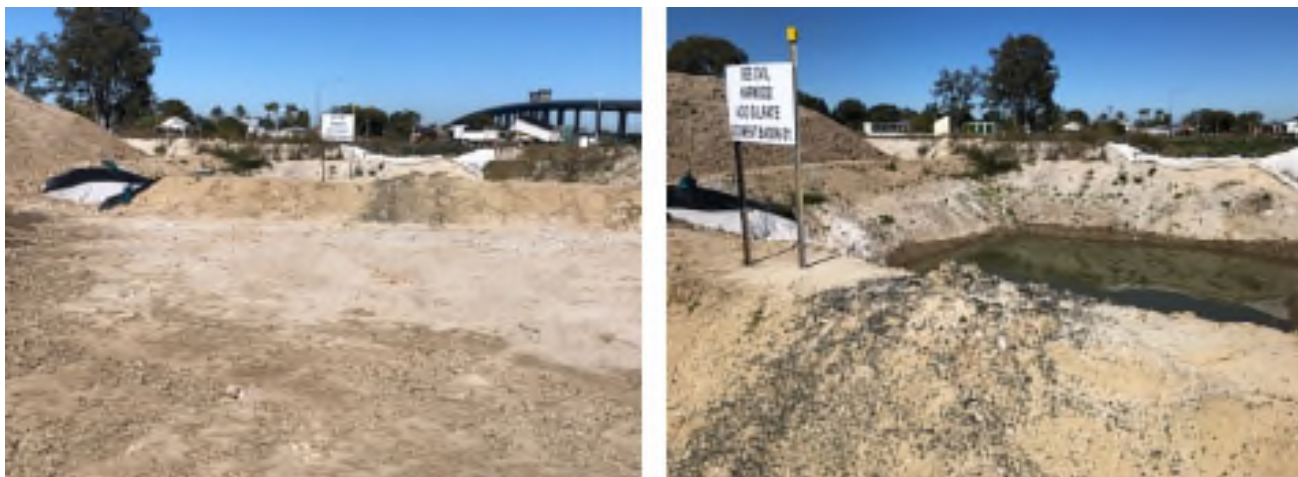
Figure 55 Harwood North ASTA sump
