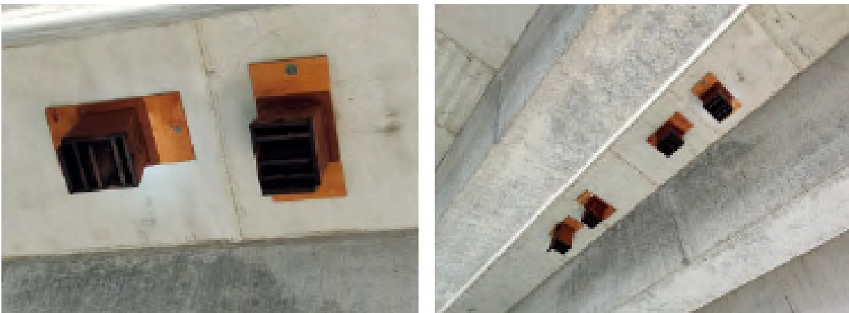
Figure 70 Microbat habitat boxes under Bridge B08
