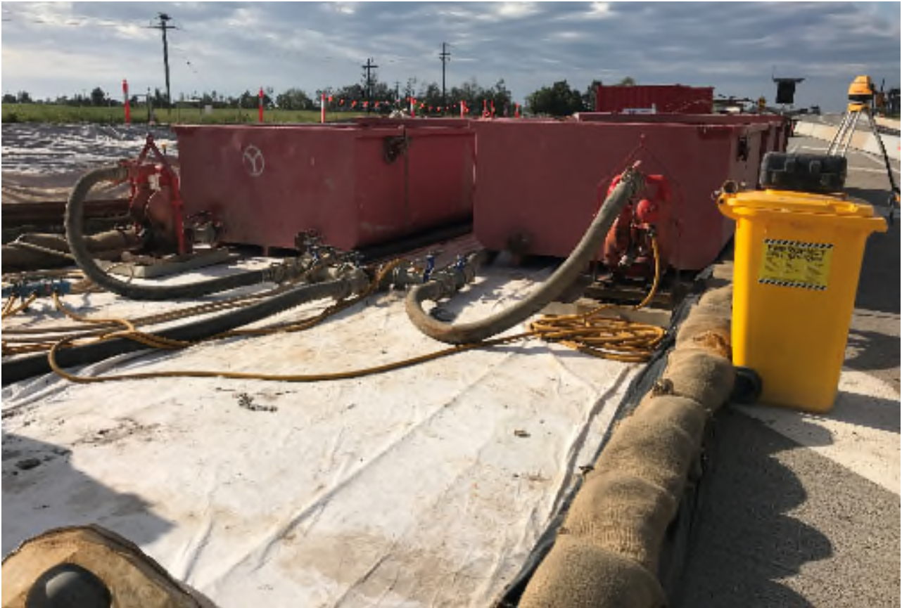
Figure 53 Bunding of a polymer tank at Bridge 68 Stage 2
