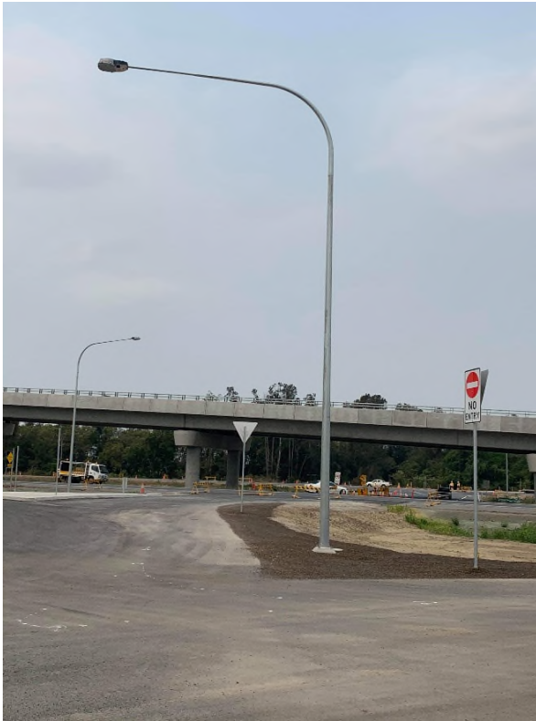
Figure 14 Street lighting installed in Section 5
