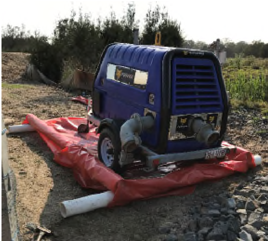
Figure 61 Innovative bunding system developed to capture any spills resulting from refuelling
