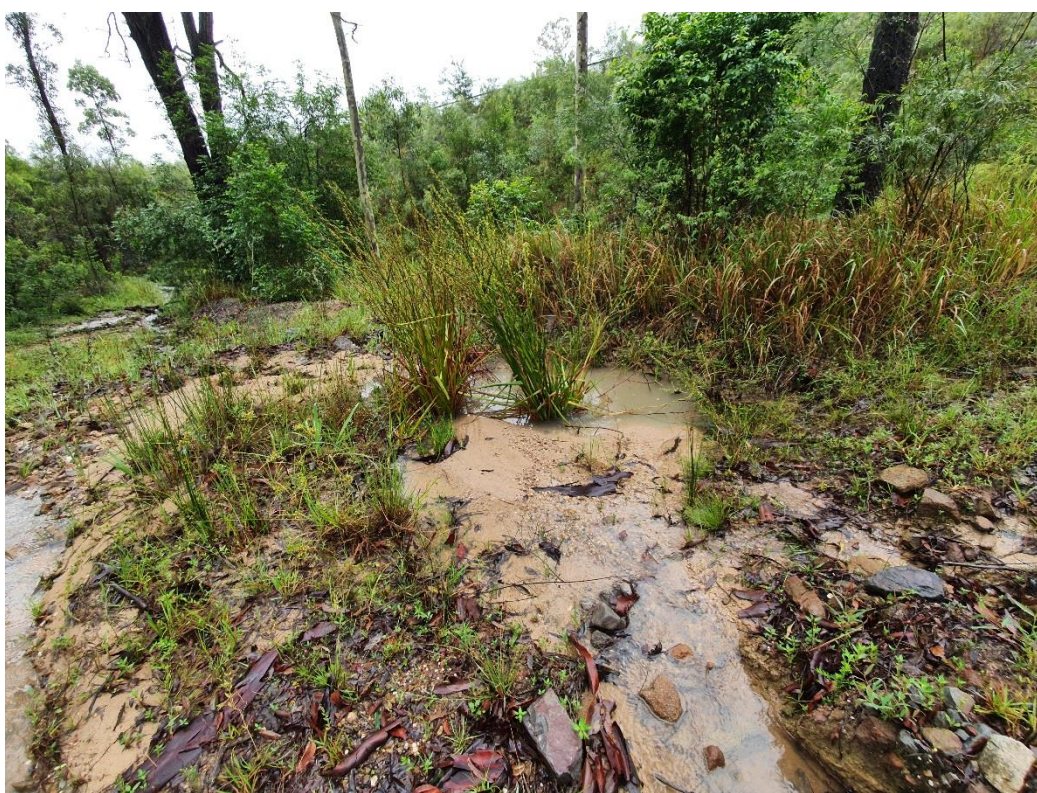
Plate 4-6. Pond inspection in mid December 2020 at Falconers (ch.11800) with some showing signs of siltation.
