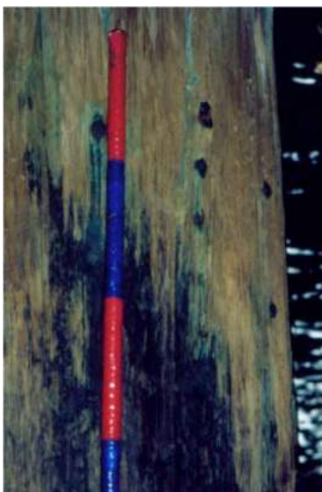
Figure 281: Sheathing tacks and copper staining on a pile from Walsh Bay 2/3. 286 Scale in 100 mm increments.
