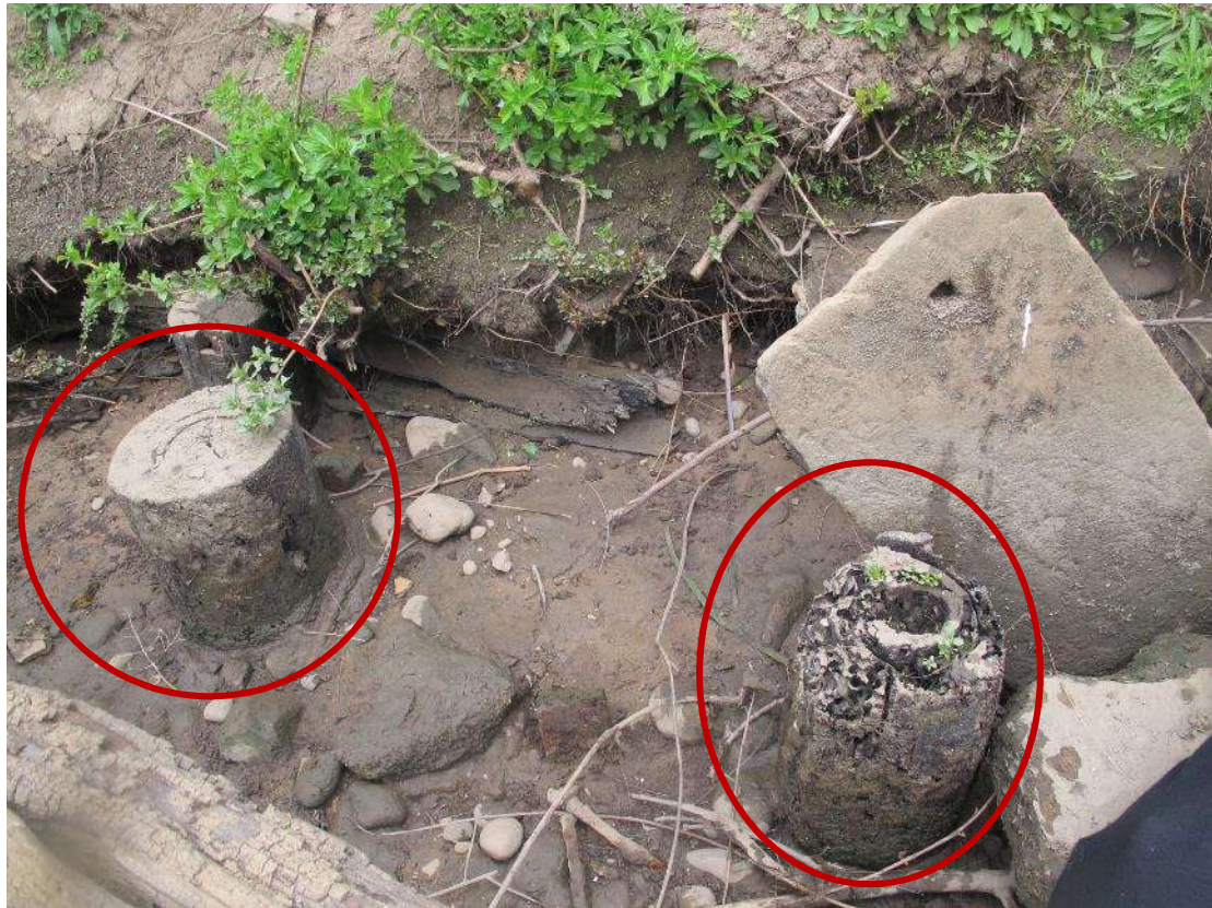
Figure 120: Cut off piles AWF6/10 and AWF6/11. Note heavily degraded pile to the right and bolts near the base of these piles.
