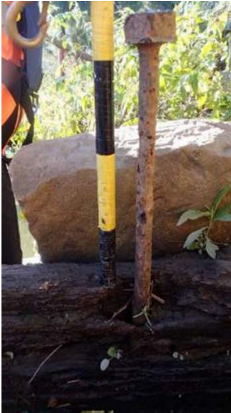
Figure 129: Through bolt joining deck beams to walers. This bolt is through waler AWF6/4 with the deck beam no longer present. Scale in 100mm increments.
