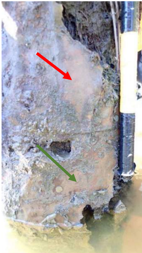
Figure 121: Remains of copper sheathing on the western side of AWF7. Red arrow indicated potential sheathing repair and brown arrow indicates sheathing lined notch. Scale in 100 mm increments.
