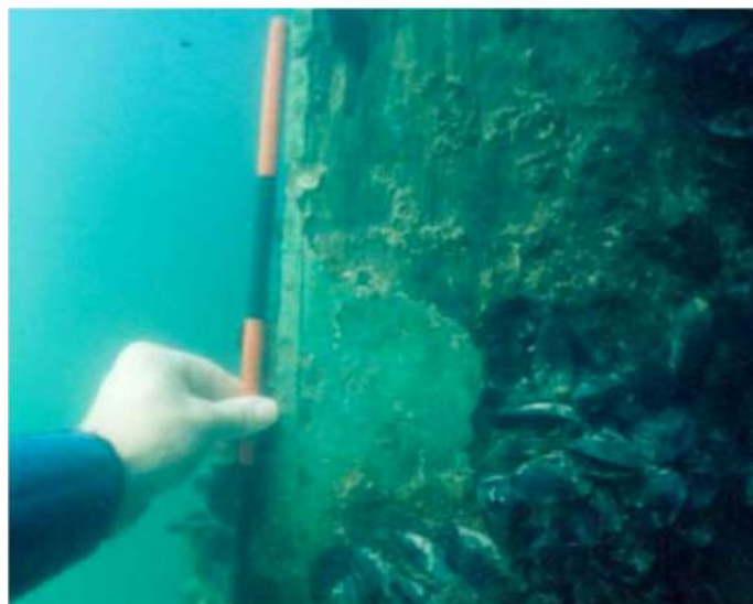
Figure 282: Remnant sheathing tacks on a pile from Walsh Bay 2/3. Scale in 100 mm increments.
