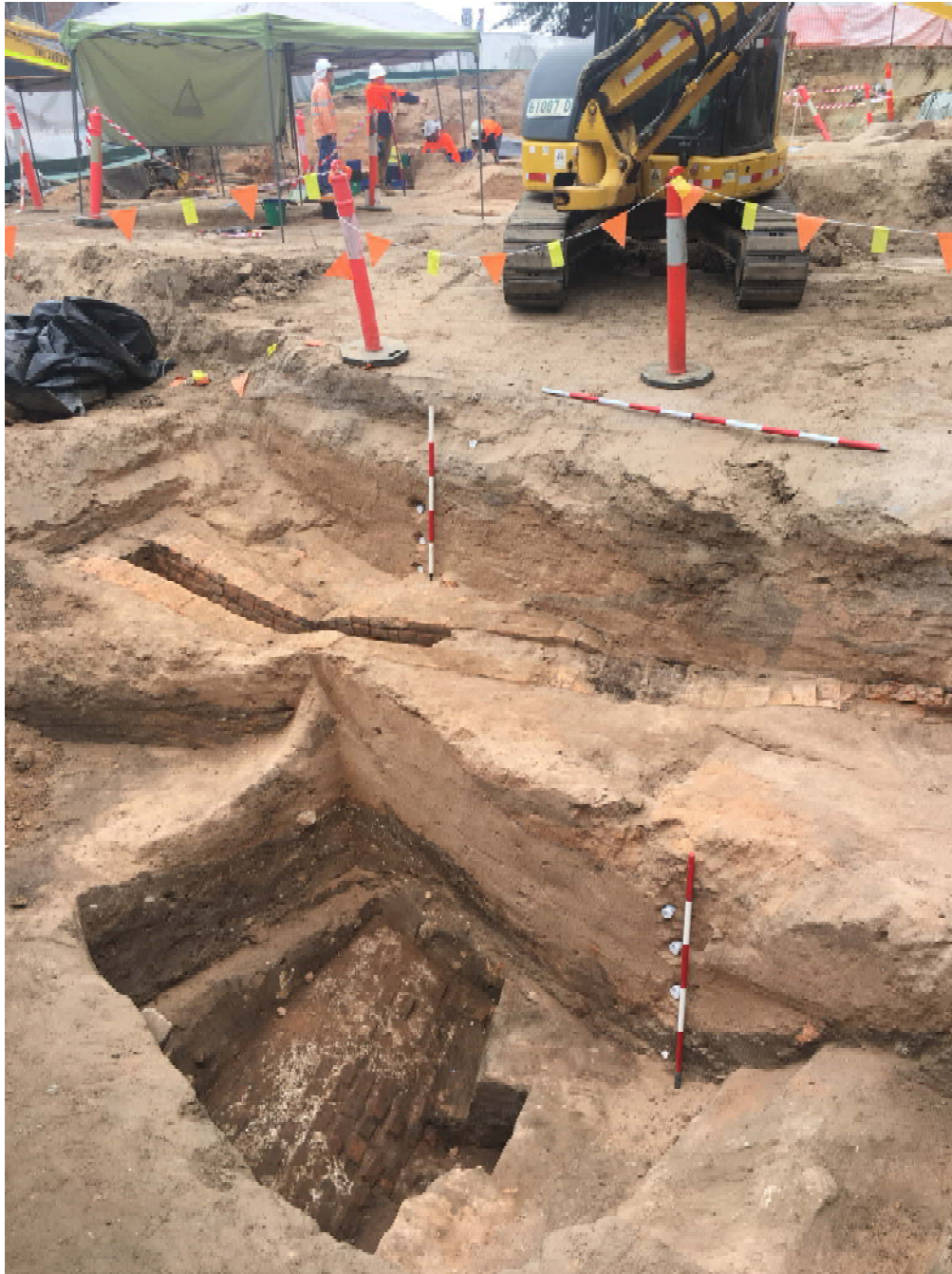
Plate 19. The northern portion of the study area, looking south. A large colonial drainage system (shown here) was found running through the study area, the installation of which required a 5-11m wide trench truncating and re-depositing the pre-colonial sand units across the site. The original trench extended the entire width of the photograph. The excavator is situated on the colonial land surface, and shows that the trench was ~2m deep in places, shallowing to the south to ~1m. Due to the trench fill being re-worked Pleistocene deposits known to contain Aboriginal objects, it was bulk excavated and sieved for cultural material. As such all material shown here – about 200m 2 or some 720 tonnes - between the people in the background to, and including sediment from, the excavations in the foreground were recovered and wet-sieved. Some 14,755 Aboriginal objects were recovered.
