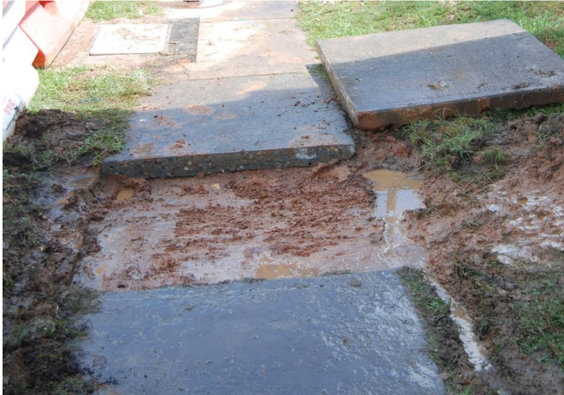
Plate 6: View north showing the footpath slab [001] removed from the trench revealing the surface of the underlying deposit [002]
