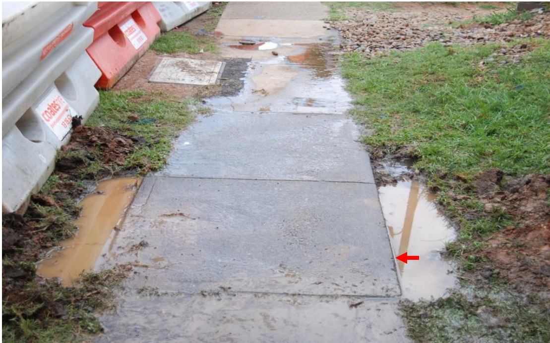
Plate 5: View north showing the slab to be removed (indicated by the arrow) for the test trench with the recent disturbance just to the north of this site caused by enlarging a service pit also visible
