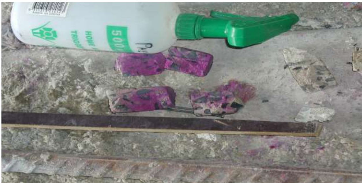
Core samples showing the extent of realkalisation of concrete (purple) in the edge beams.
