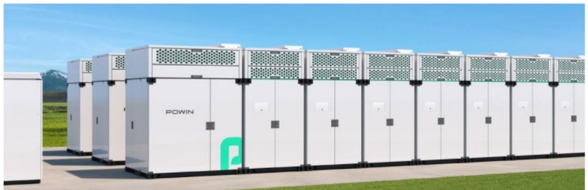
Figure 3 | Example of a battery storage cabinet
