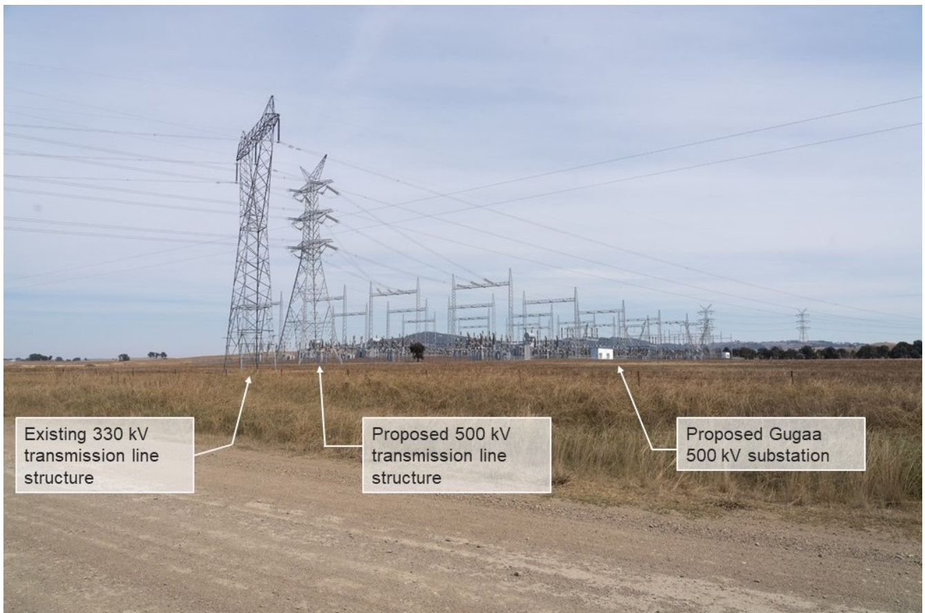
Figure 3-6 Photomontage of the proposed Gugaa 500 kV substation looking south from Livingstone Gully Road
