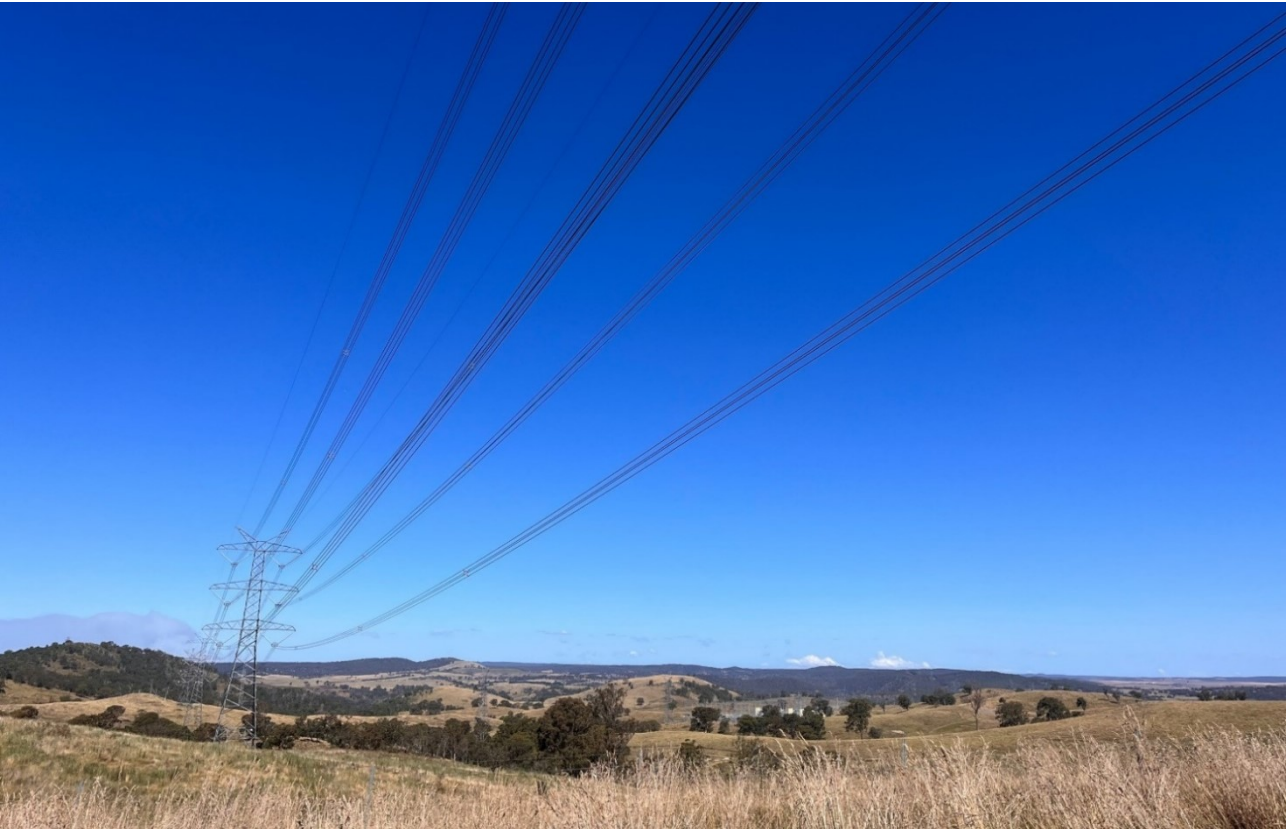
Figure 3-3 Example of 500 kV transmission line structures
