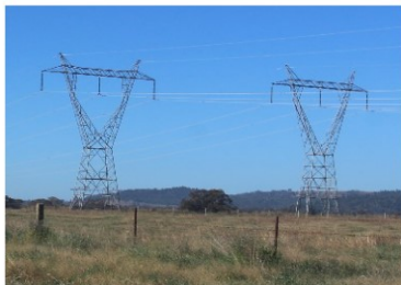
Tall and wide steel lattice
