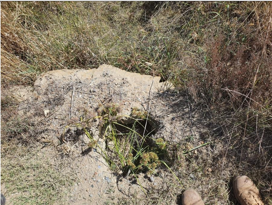
Partially blocked upstream culvert
