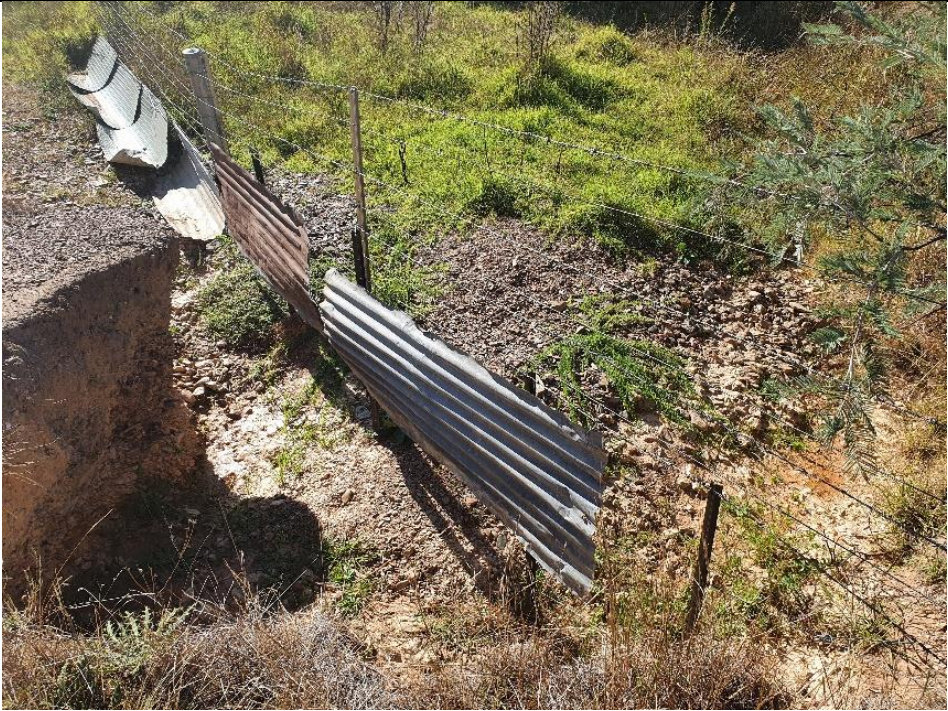
Informal fencing structure
