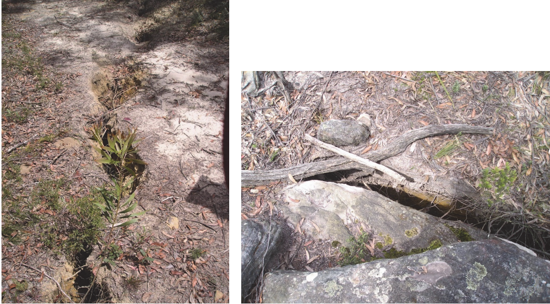
Fig. 5.19 Surface tension cracking due to downslope movements at the Dendrobium Mine
