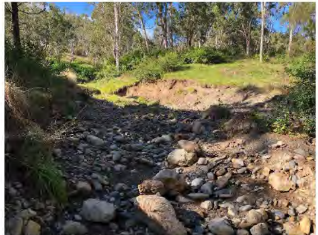
Plate 7.9 Example of high energy flood damage observed in various areas across the Project area, view south east
