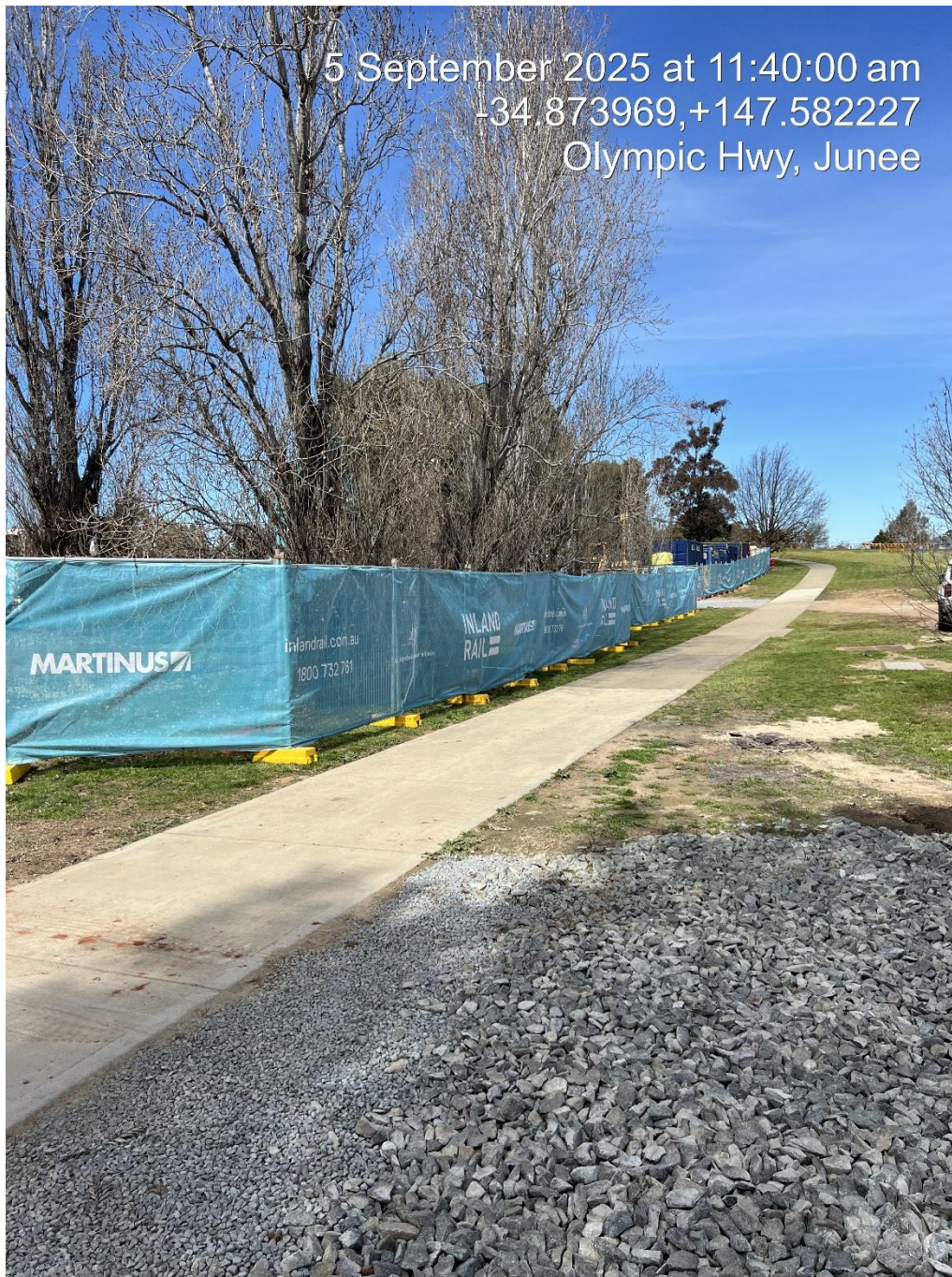
FIGURE 8 Rail exclusion fencing in place on the western side of the rail corridor looking south from the existing boundary fencing along Seignior Street
