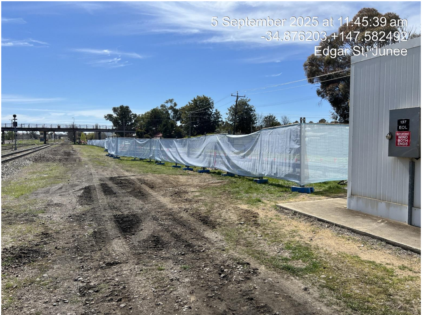
FIGURE 6 Rail exclusion fencing in place on the eastern side of the rail corridor extending north from William Street along Edgar Street
