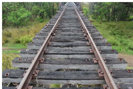
Figure 5-10: Example of the railway line along the approach to the Gwydir River Underbridge, view north-east. Source: Artefact Heritage
