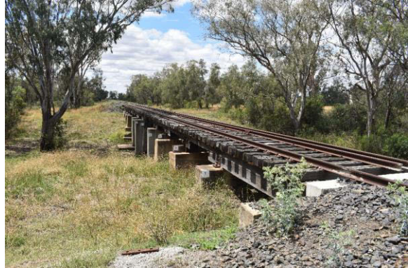
Figure 4-12: The 14 span timber and concrete constructed underbridge over Skinners Creek at Chainage 667.945
