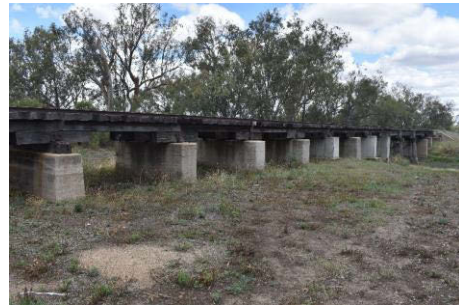
Figure 5-12: Example of underbridges along the railway line over Duffy's Creek. Source: Artefact Heritage
