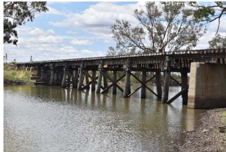
Figure 5-11: Example of underbridges along the railway line over Skinners Creek. Source: Artefact Heritage
