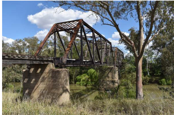
Figure 4-8: The Camurra, Gwydir River Underbridge from the north bank of the river
