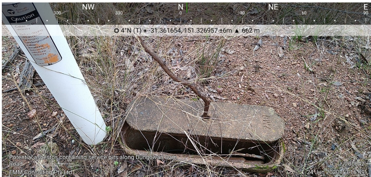
Plate 9 Potential asbestos containing service pits along Dungowan Dam Road
