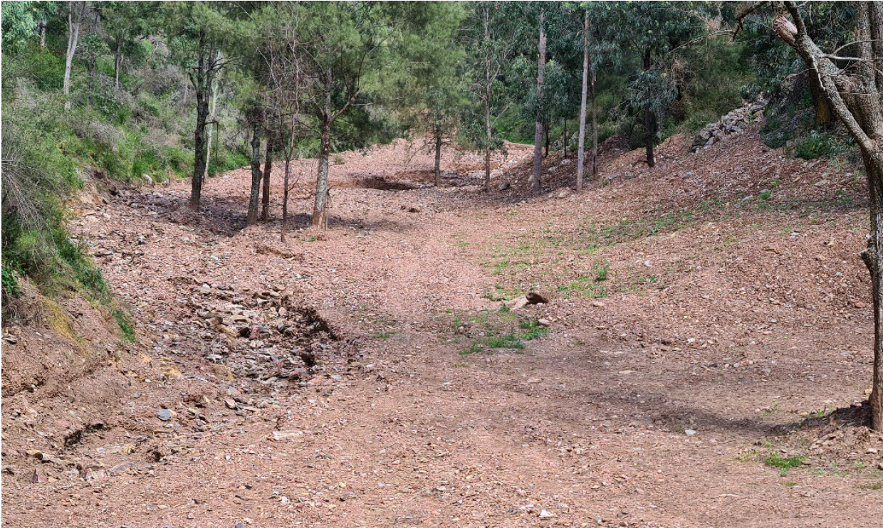
Photograph 13-1 Existing erosion hazard observed in a lateral gully that feeds Dungowan Creek
