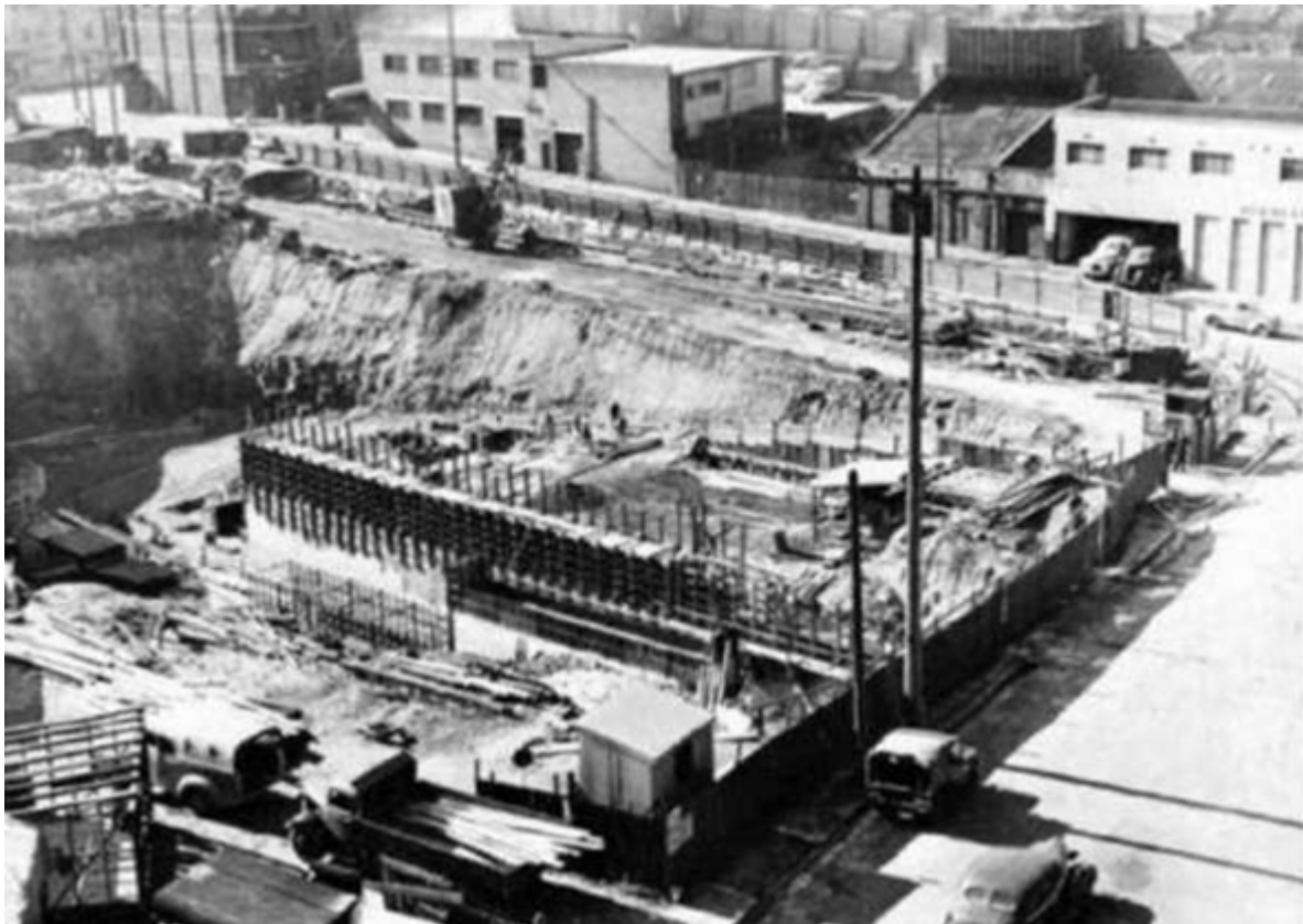
Figure 5 Historic photo showing excavation associated with the Eastern Suburbs Railway (Source: Unknown)
