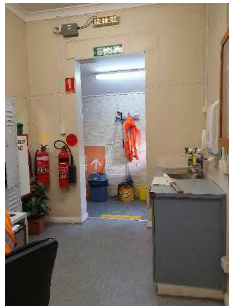
Figure 70 Electrical room shows the conversion of the former toilets and lean-to structure beyond
