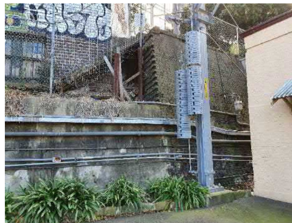
Figure 55 Termination of the original retaining wall at No. 125 Little Eveleigh Street and adjacent Store Building
