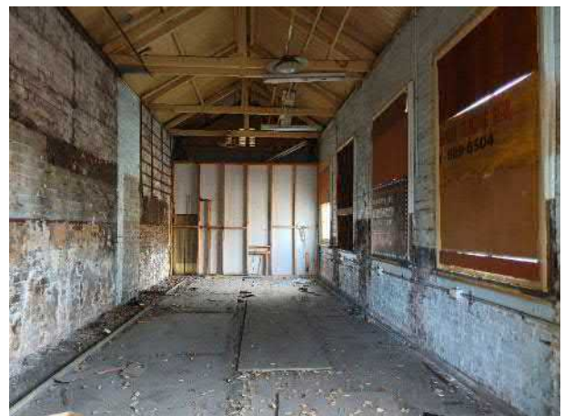
Figure 51 Interior of the principal building showing rare exposed timber trusses and timber panelled ceiling.
