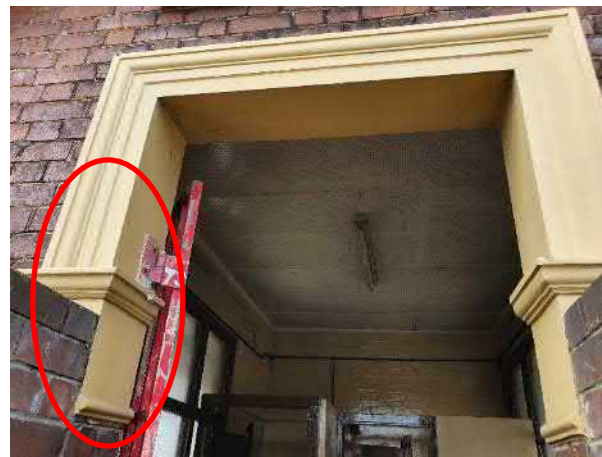
Figure 66 Entry to male toilets showing blade walls over mouldings
