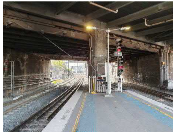
Figure 39 Lawson Street overbridge showing a combination of jack arch, steel girder and concrete slab construction
