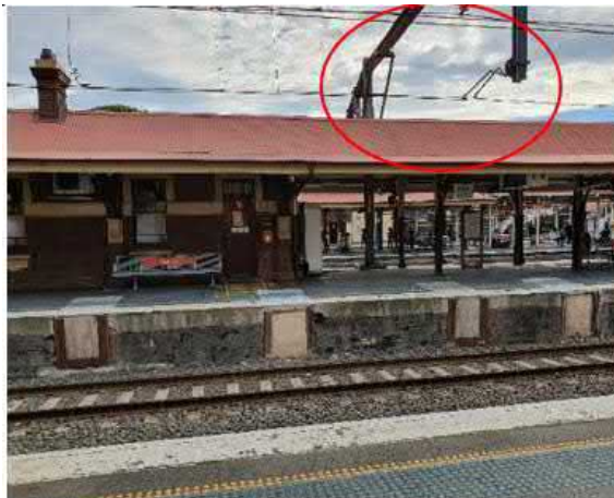
Figure 73 OHW structure SWI+267
