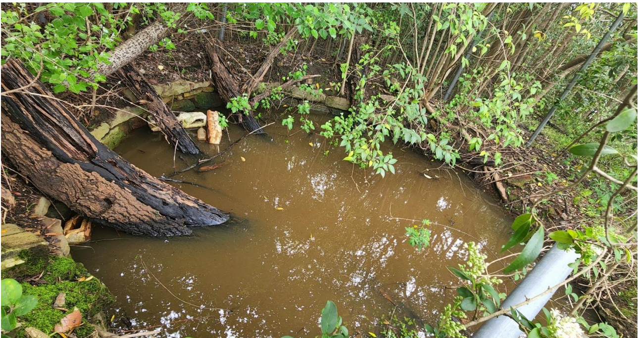
Figure 6-41: The large stone well or cistern on inspection in 2022 at which time the fence was partially damaged, and the well, full of water
