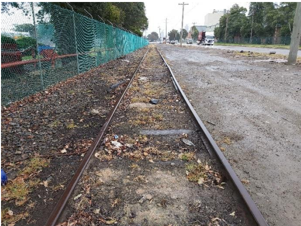
Figure 6-3: Tram lines along Grand Avenue, Camellia that are part of Parramatta LEP 2011 Item I6
