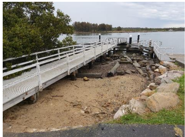
Figure 6-38: Wharf remnants adjacent to Ermington Boat Ramp, Melrose Park demonstrating the environment in the area.
