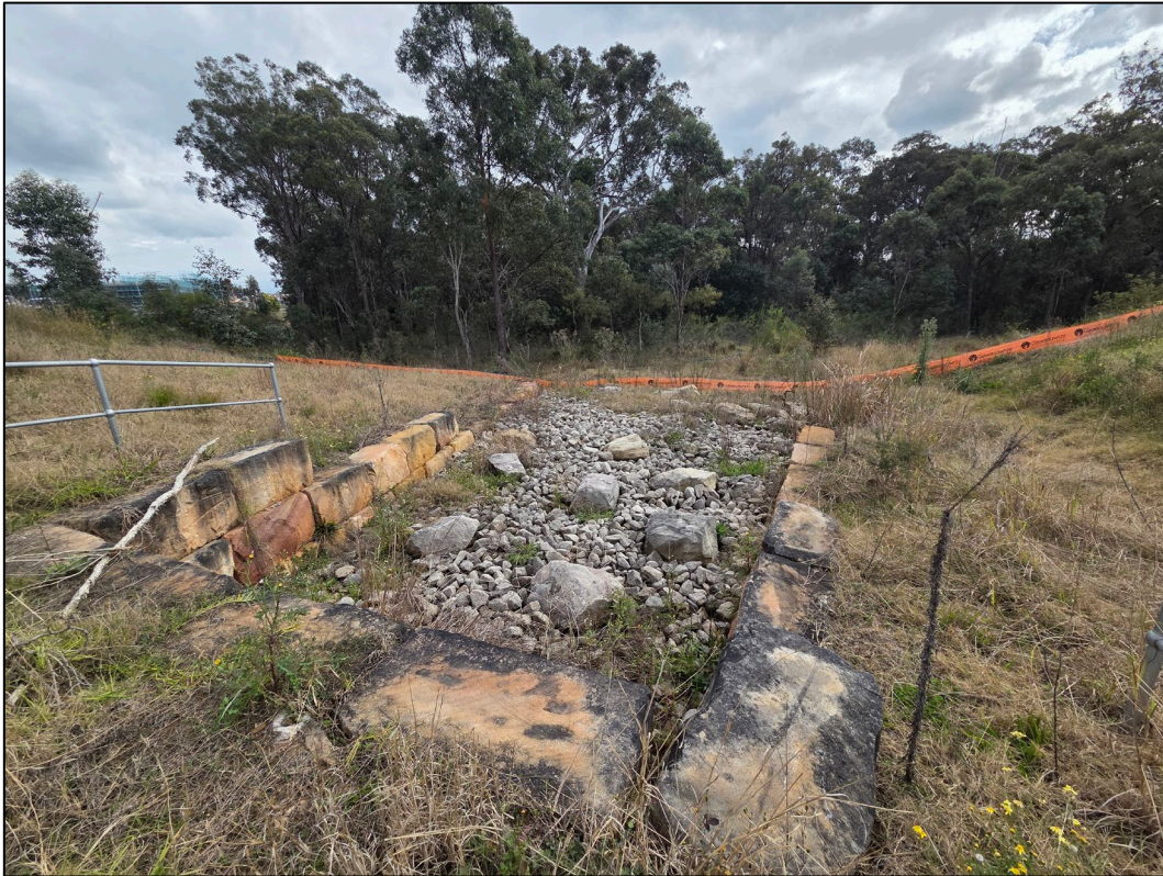
Site Photograph 6.2.2 View of the sandstone drainage culvert within Lot 9 in DP1275478 (north of Buchan Avenue), as observed facing west on 8 August 2025.
