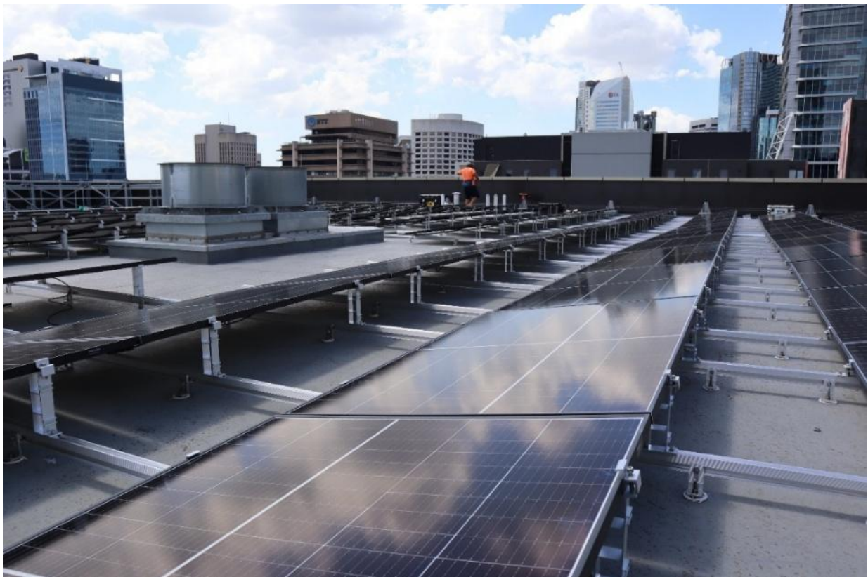
Figure 5 PV Solar on Roof
