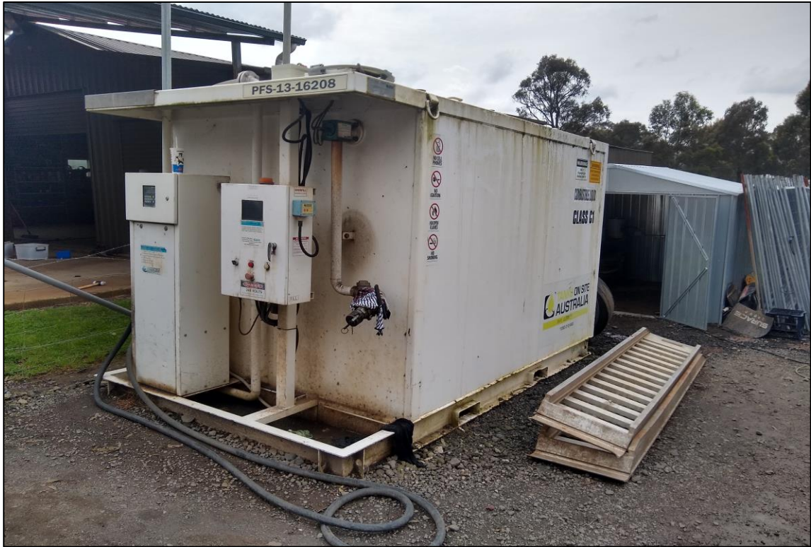
Photograph 01 A portable toilet unit located at the site of the investigation. The unit is a white, rectangular structure with a control panel and a black hose. It is situated on a gravel surface next to a building.
