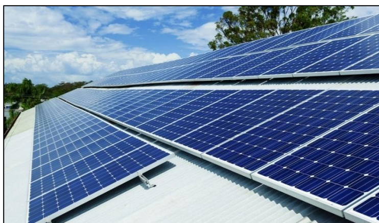
Figure 5 Rooftop Solar PV (Source: Google images)
