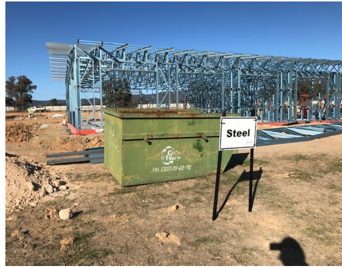
Photo 6 – Steel waste bin.
