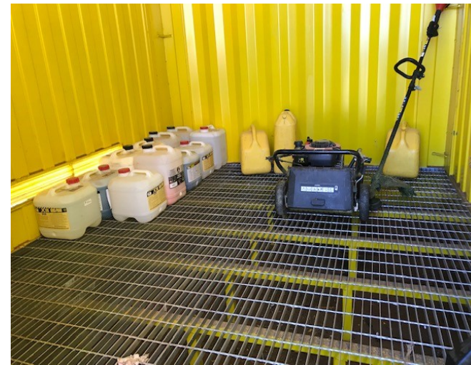
Photo 8 – Bunded chemical container.
