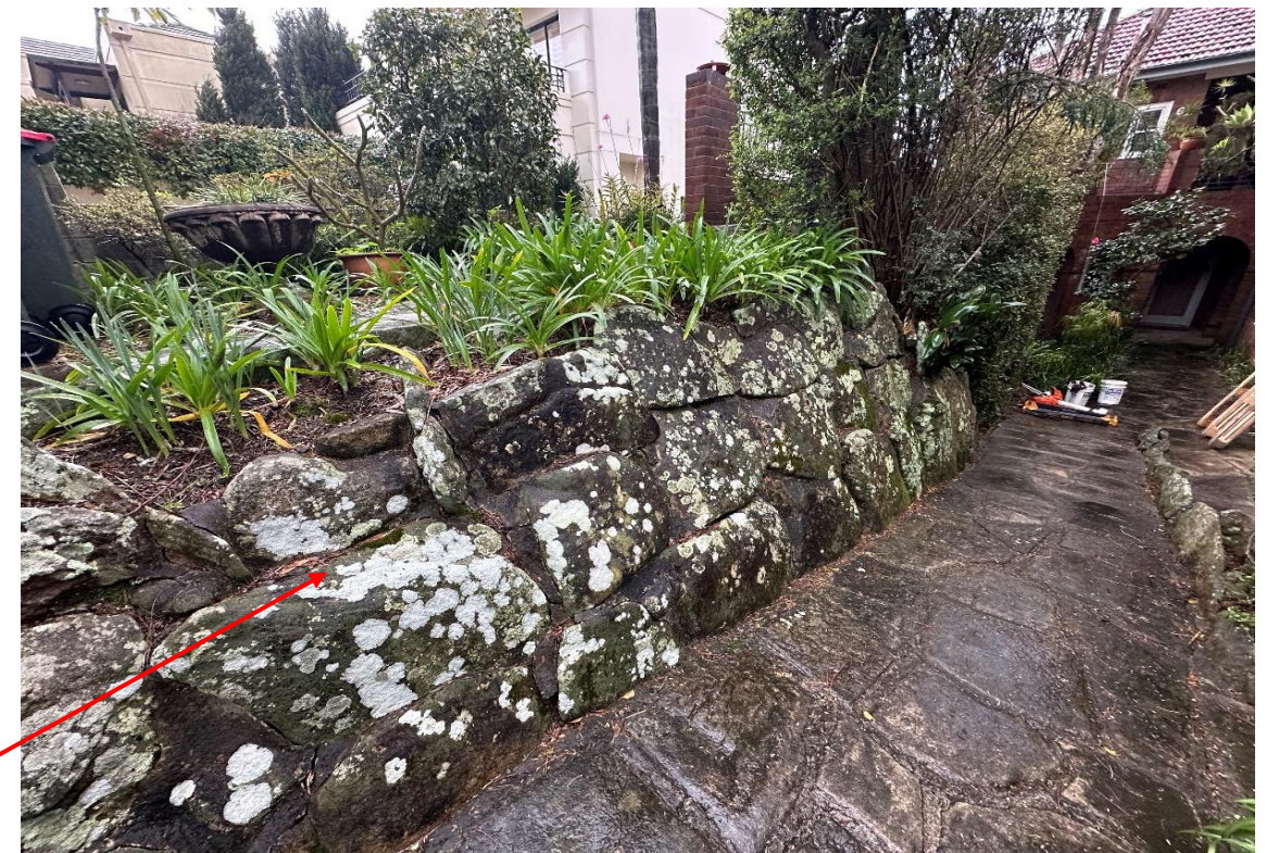
Photo 6: Bulging garden bed retaining wall
