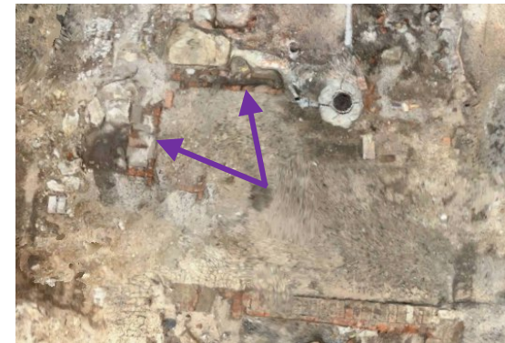
Figure 24: 1025 and 1028 with associated contexts with 1028 shown at top of image with drain.
