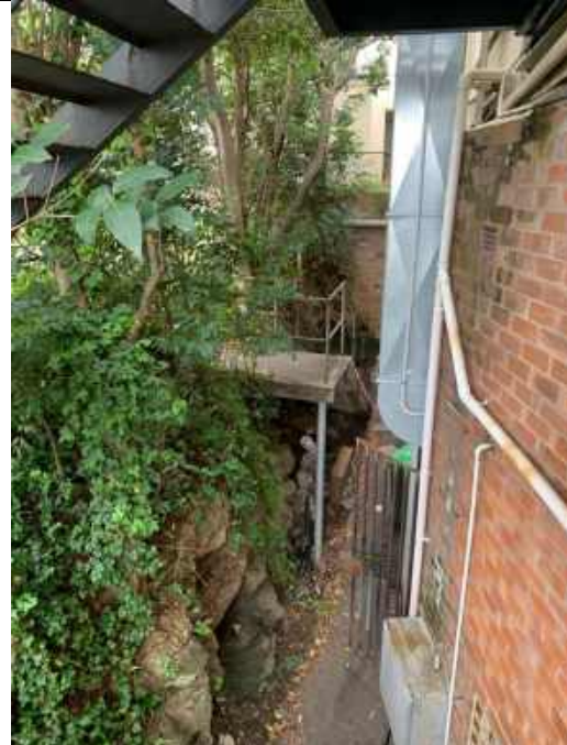
Plate 4: view of the basement access at the rear of the commercial building
