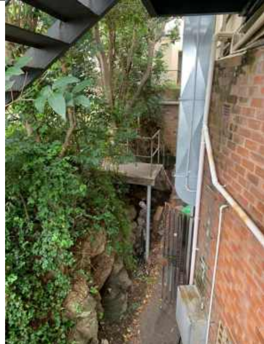
Plate 4: view of the basement access at the rear of the commercial building
