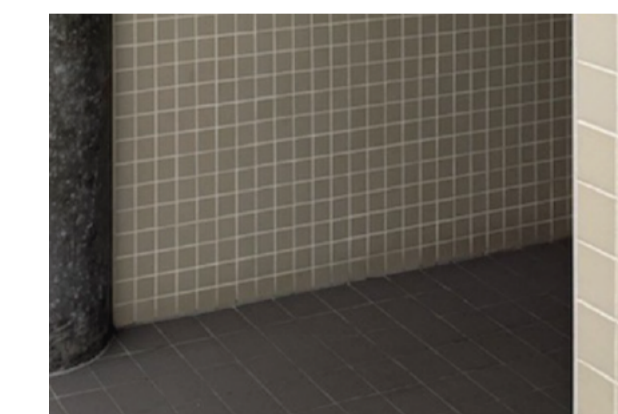
Ref image - Site conditions 100 x 100 floor and wall tiling to match adjacent Male WC, as fitted beyond the entry Vestibule in 2021
