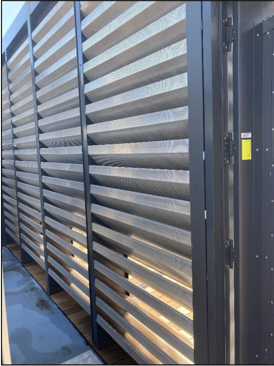
Figure 10 – Noise softening panels, rooftop HVAC area
