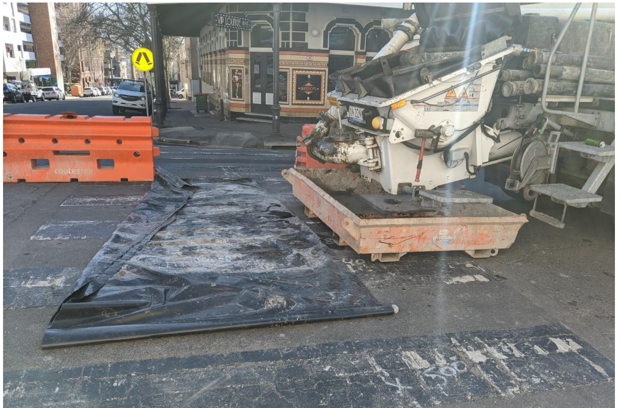
Concrete washout observed during conduct of the site inspection on 26 August 2020. Church Street
