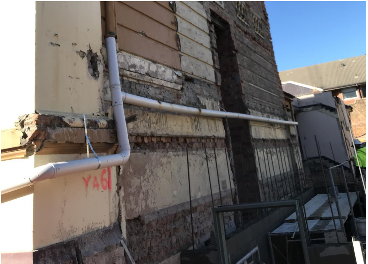
Piping used to divert clean water captured from on-site to existing Council stormwater drainage.
