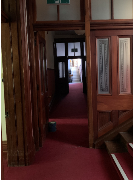
Figure 5 | Existing Doorway Circulation Obstructed by Stair
