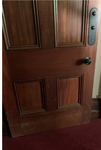
Figure 6 | Existing Doorway with non-compliant handle
