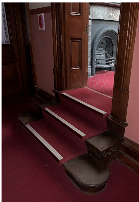
Figure 2 | Existing Stair Protrudes into Corridor
