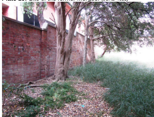
Plate 21: Tree roots damaging the southern wall. (4606)
