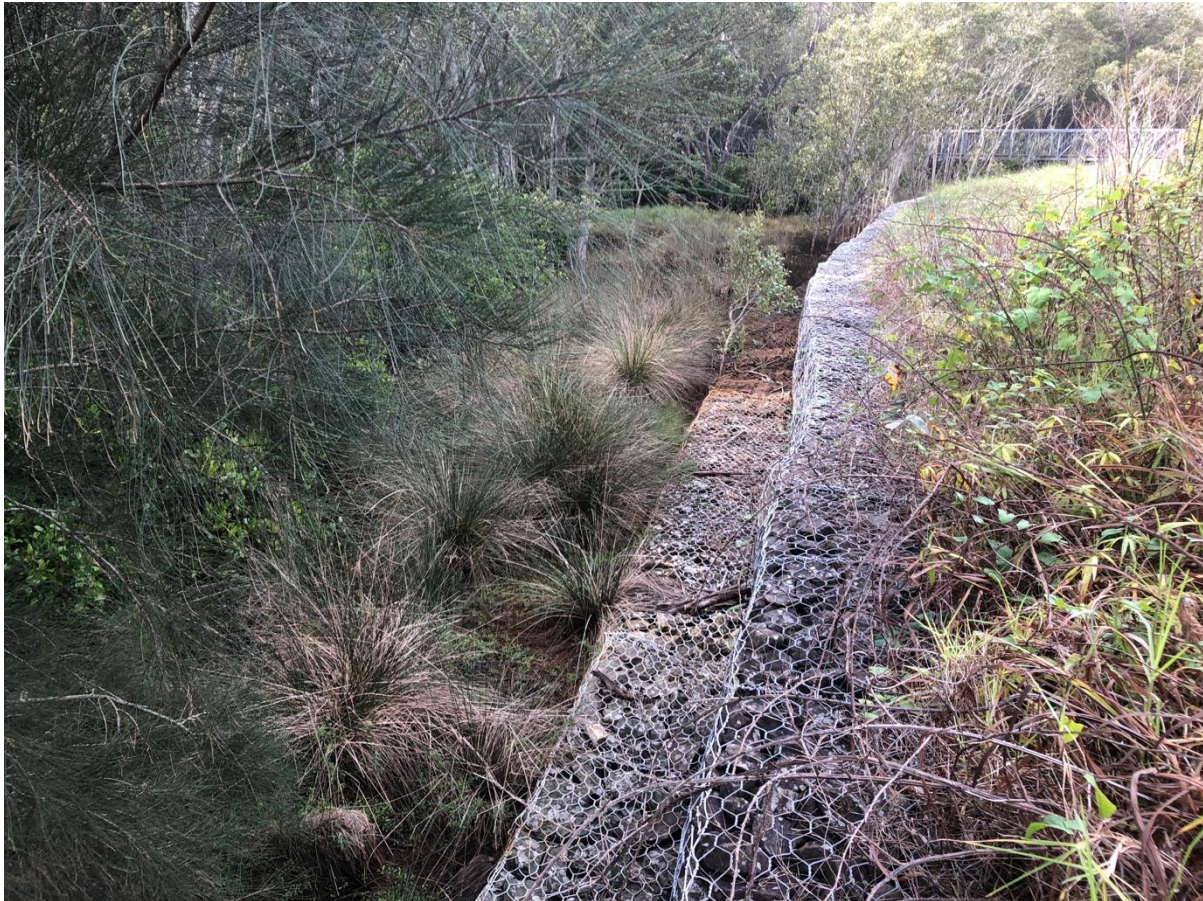
Photo 7 – Edge of Stringybark Creek showing gabion wall containing the contaminated fill lands – top of bank for Stringybark Creek coincident with the wetland vegetation boundary
