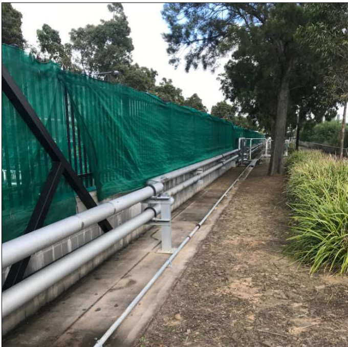
Figure 7: Infrastructure associated with the Botany Groundwater Clean-Up Project along the southern site boundary (Source: Keylan Consulting)
