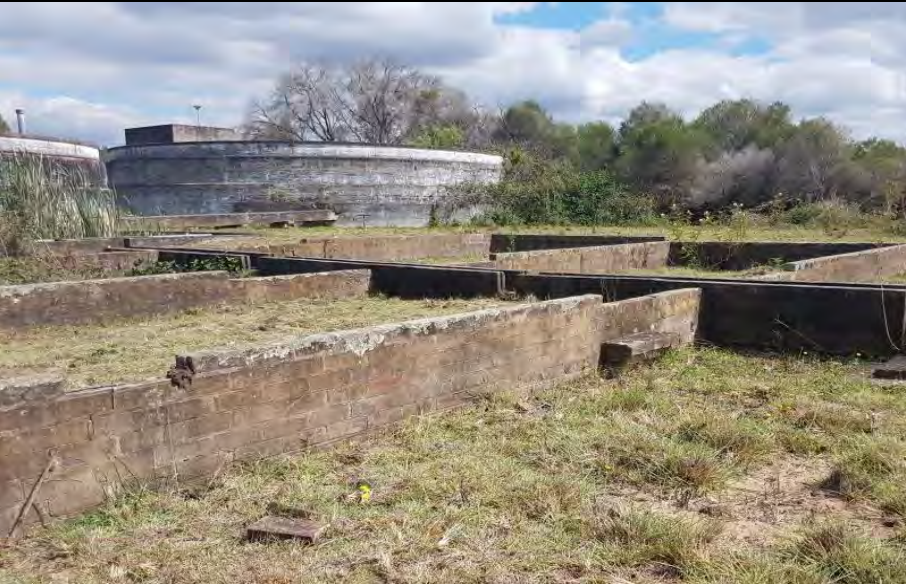
Photo 11 WWTP Sand Filter
