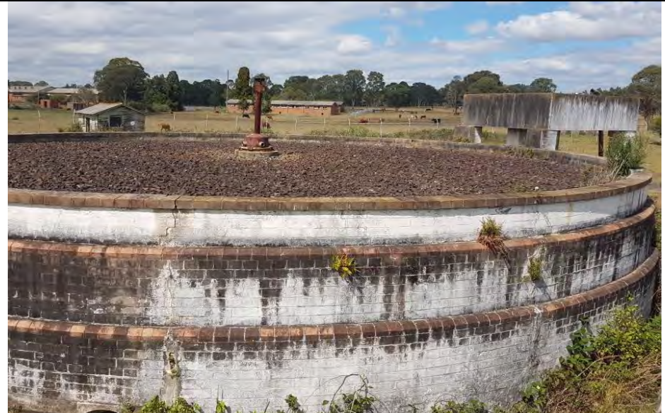
Photo 12 WWTP Aerobic Treatment Tank with Rock Bed
